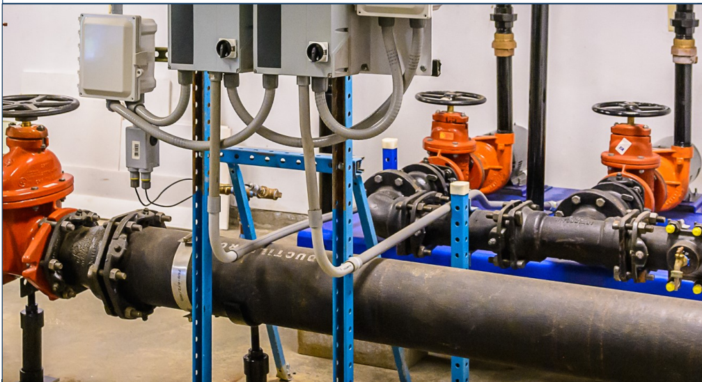
Pumps and valves in Well House #3.
